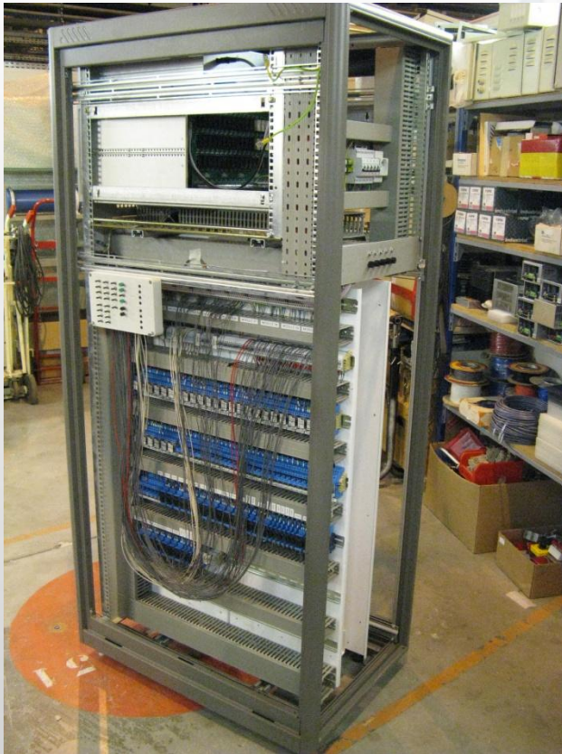
Central cubicle of SSRT patient safety system during initial testing
