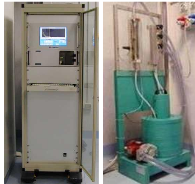
Air/Gas monitoring system
